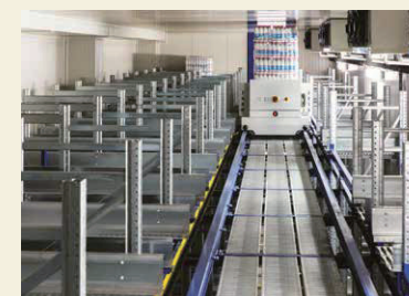
ASRS - Automated Storage & Retrieval System
